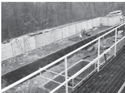
The workers are heat sealing the liner in the new sediment tank, which will hold the backwash. Compare the size to the small concrete tank shown on the right that is in use now.
